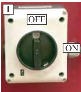
1 MAIN ISOLATING SWITCH
